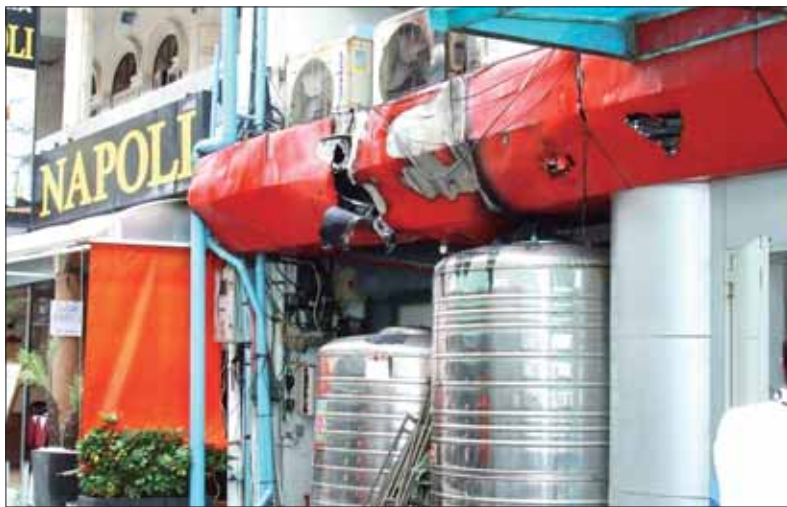
A fire broke out last November in Patong when an air compressor shorted.
