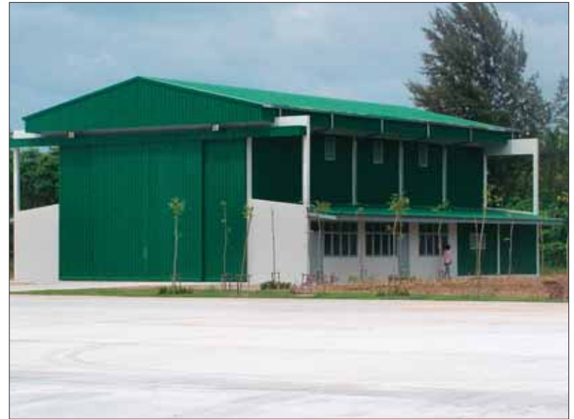
HANGING IN THERE: A helicopter hangar at the new site of the Police Region 8 headquarters, currently under construction in Mai Khao.
